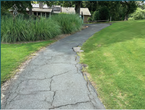
A typical golf cart path requiring attention
