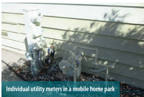
Individual utility meter hookups in a mobile home park
